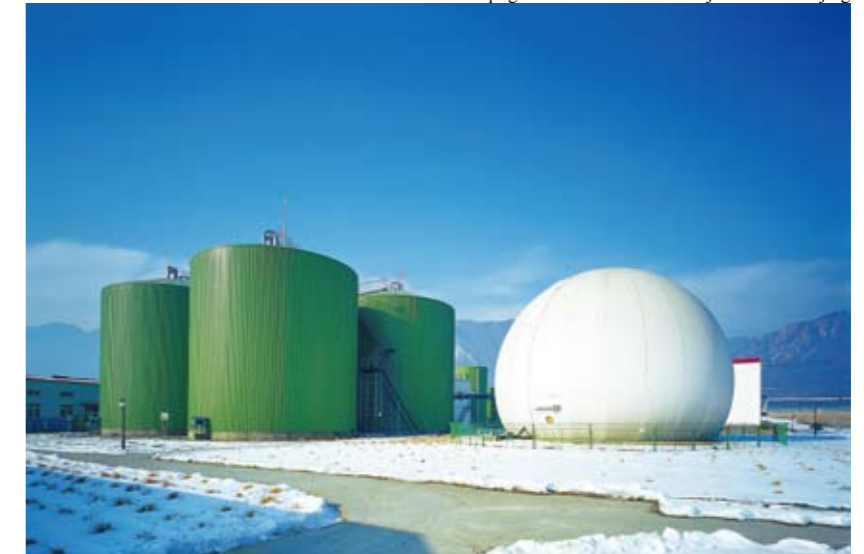
● Yanqing 2 MW Biomass Gas Project Site in Beijing
