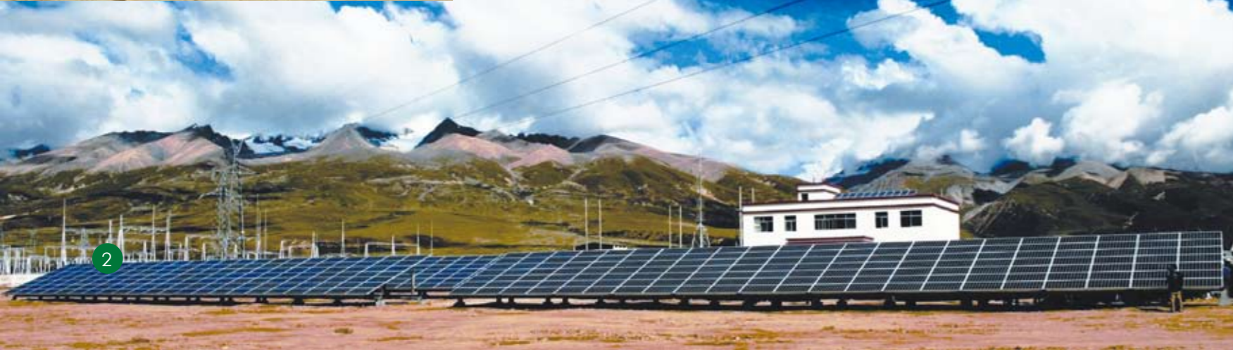
● Yangbajing High Voltage Grid-Connected Photovoltaic Power Plant in Tibet
