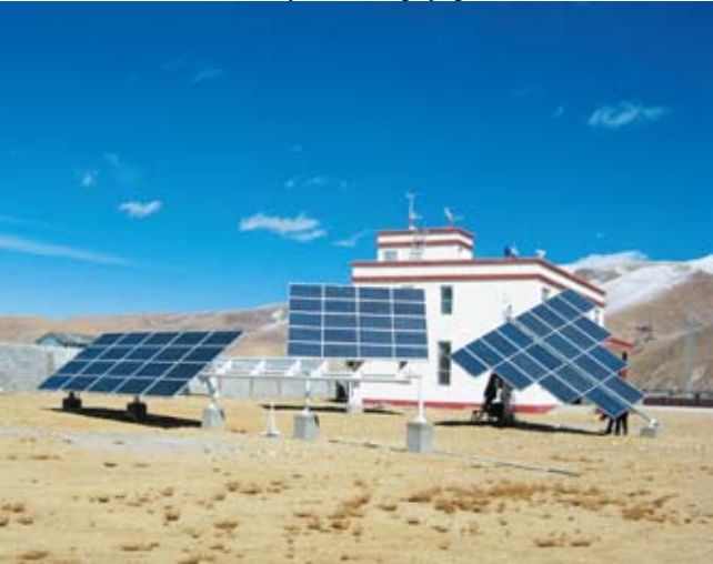
● Multiple Photovoltaic Automatic Tracking System in Yangbajing in Tibet
