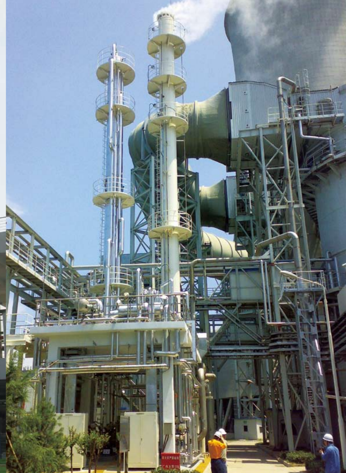
● 120,000 t/a CO 2 Capture Project in Shanghai
